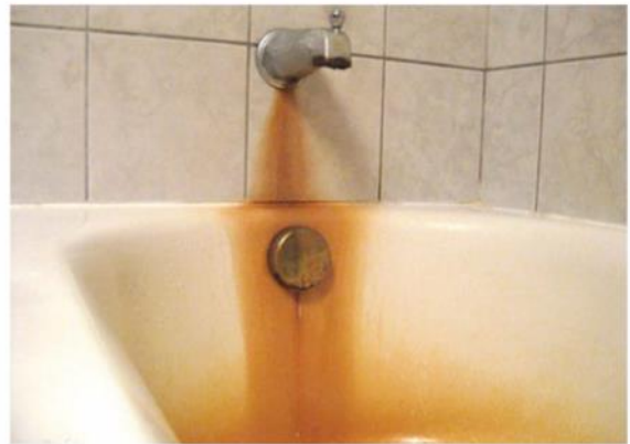
Image of iron staining.
