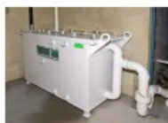
Elevator Sump Pump Interceptors
